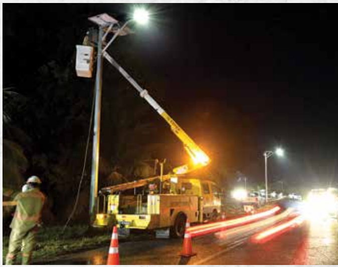
A crew from the Public Lighting Department makes final adjustments to one of the solar LED street lights installed along the Manzanilla/Mayaro Road prior to their commissioning in July.
