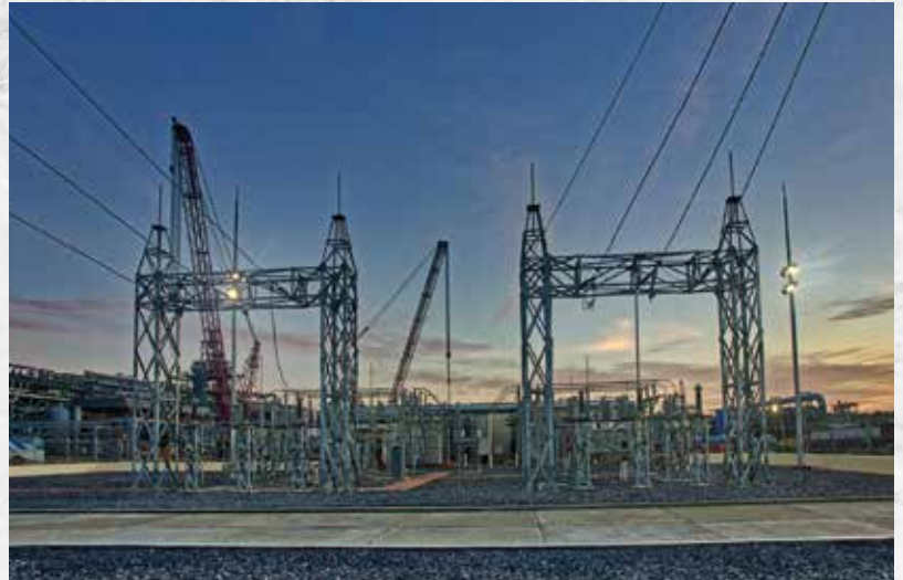
The Caribbean Gas Chemical Limited's 66kV Substation, commissioned in February, was built to provide the CGCL's methanol/dimethyl ether plant with its 16.8MVA power requirements.
