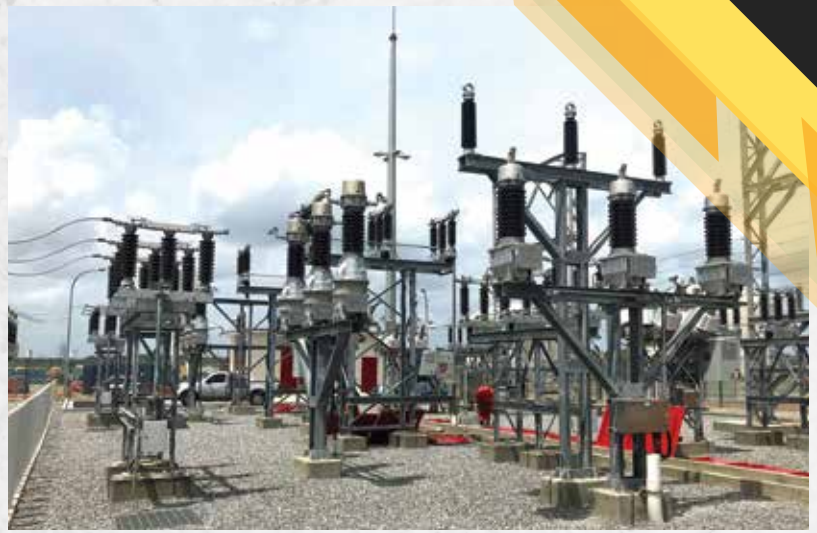
The new DeNovo Energy 66kV Substation in Point Lisas was completed in June to provide the new natural gas processing plant, DeNovo Energy Block 1A Limited, with 4MW of electric power.
