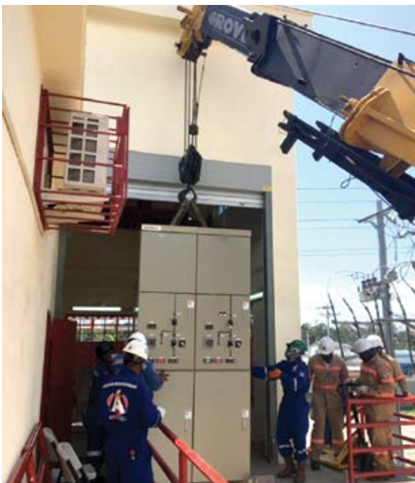
Workers spotting the Hyundai 33kV GIS Switchboard in the new switch-house at Laventille Substation.
