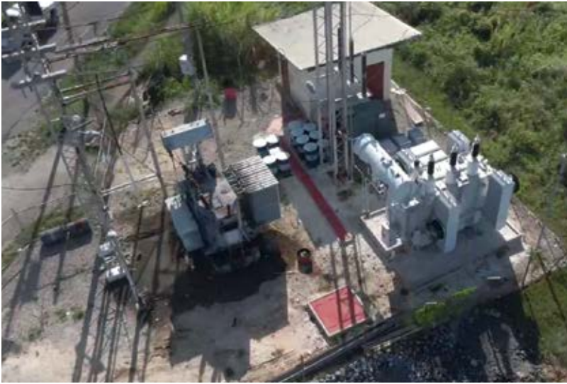
New and old transformers at Chaguanas West Substation.
