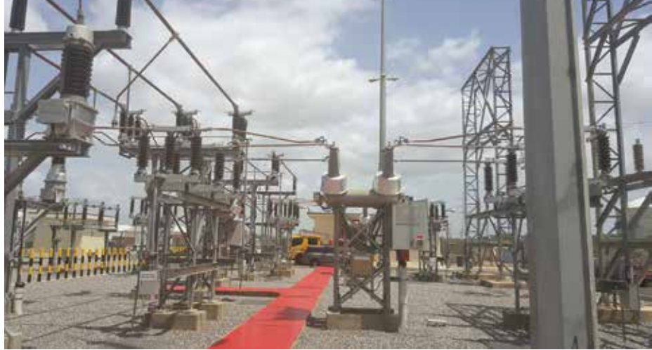
The new DeNovo Energy 66kV Substation in Point Lisas.
