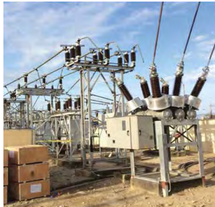
Transformer accessories to be installed on the new transformer.
