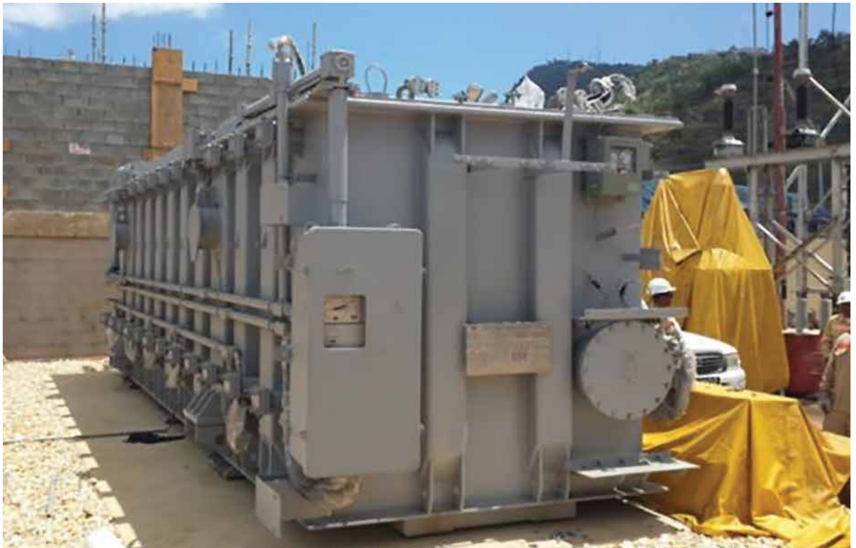
New 66/33 kV, 100/130 MVA transformer installed on the new plinth in Westmoorings Substation
