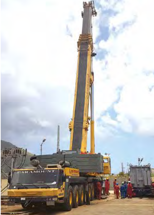
Workers prepare to manoeuvre heavy equipment to hoist the new transformer into position.
